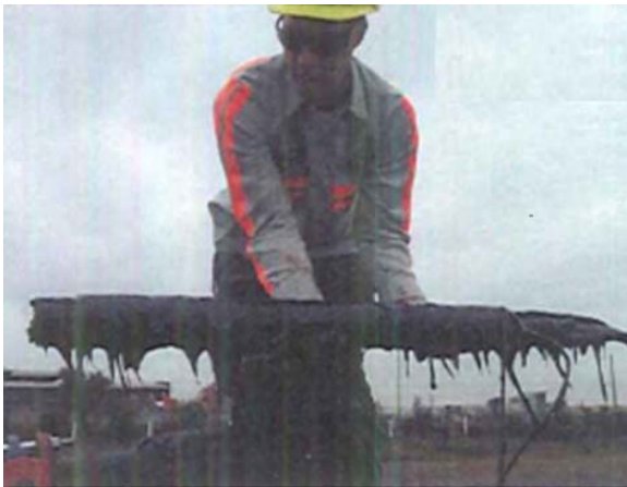
Air-powered Remediation Pumps
